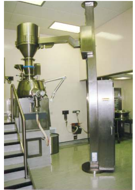
Drum Hoist with manual clamping and powered inversion. Loading a mixer granulator with a drum hoist
